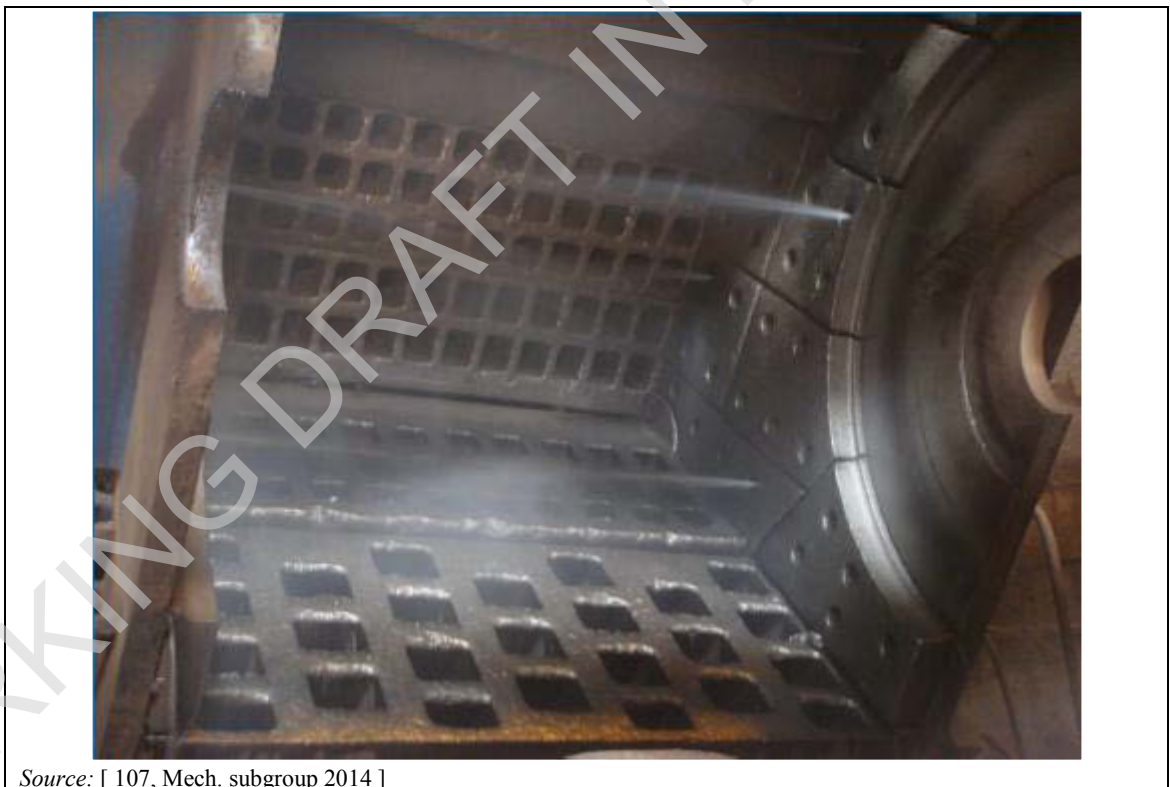
Figure 3.19: Water injection into the mill
